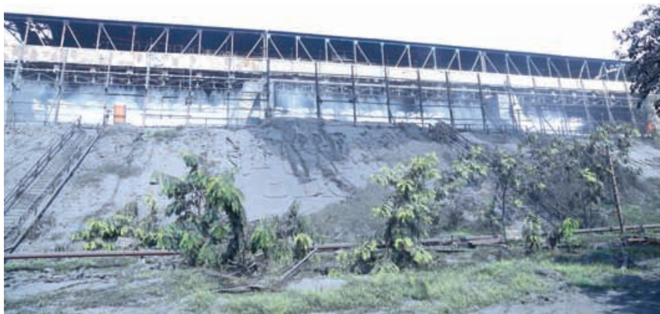
Dust suppression activity with Mist & Dry fog system at 16000 tonnes GL bunker, RG OC-3 CHP
